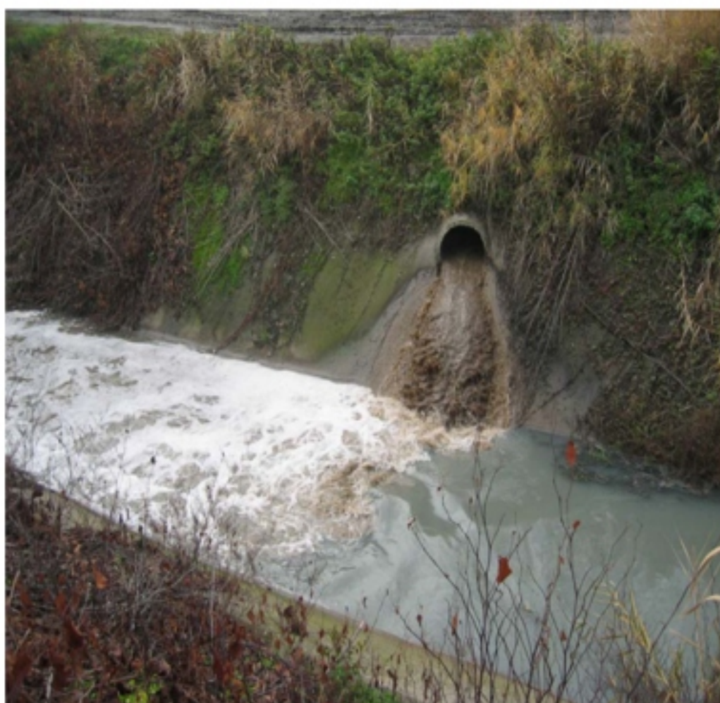
Industrial effluents are discharged untreated via I-64 lateral into the DTD-Canal
